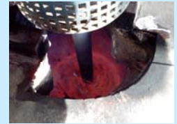
Furnace in Purging Process
