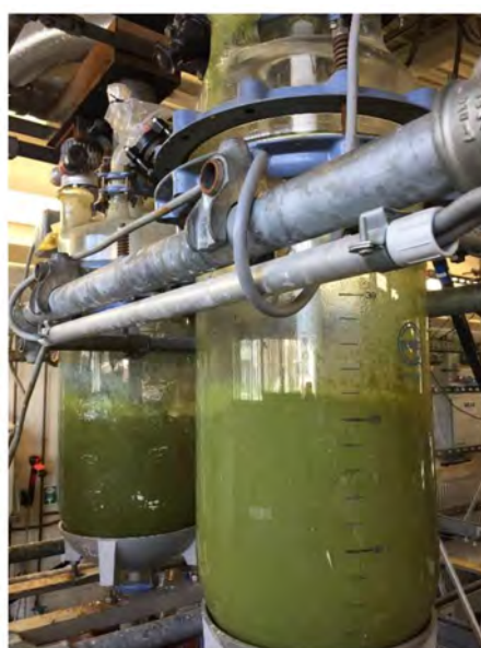
Figure 14. Treatment of eudialyte concentrate in two reactors at the Institute of Process Metallurgy and Metal Recycling (IME) demonstration plant, RWTH Aachen.
